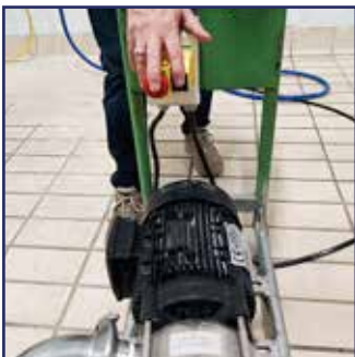
Step 10 Start the pump to draw in water to dampen the filter pack for about 3-4 minutes.
