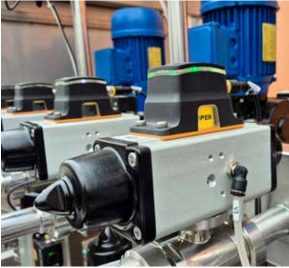
N. 14 PNEUMATIC VALVES each with an actuator and proximity sensor
